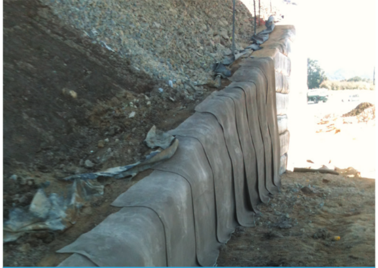
CC5 was cut to length on site to match the varying height of the abutment
