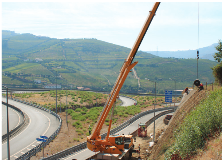
The CC was mounted onto a spreader beam and hung from a truck crane
