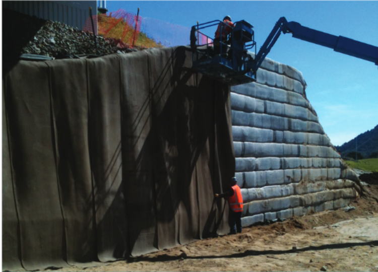
A cherry-picker was used to lift sections of CC to the top of the slope
