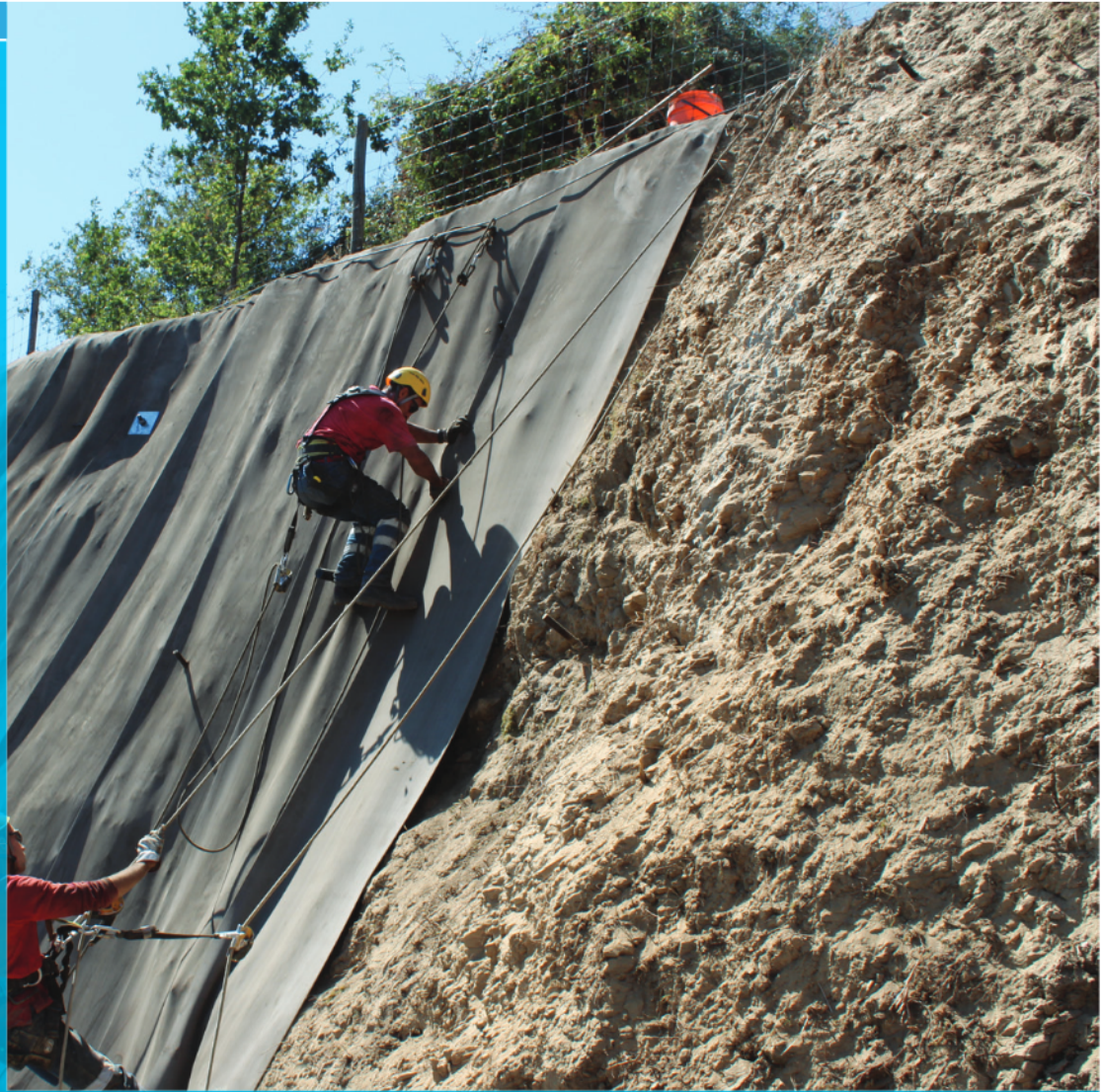
The installation team at Highway A24 had to use climbing equipment due to the restricted access of the site
