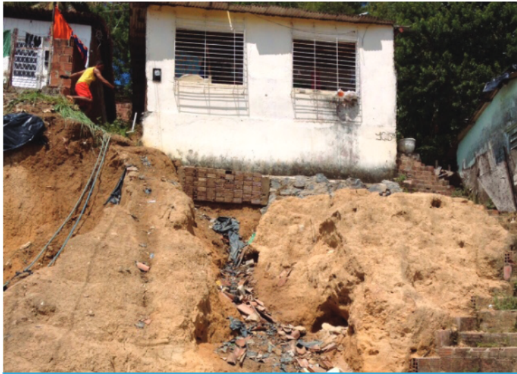
Extensive erosion of the slope
