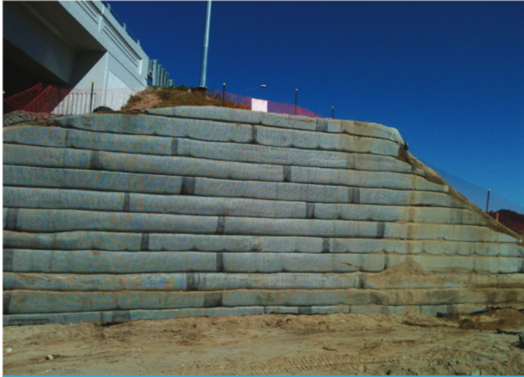
The abutment had been prepared with a geogrid prior to installation of CC
