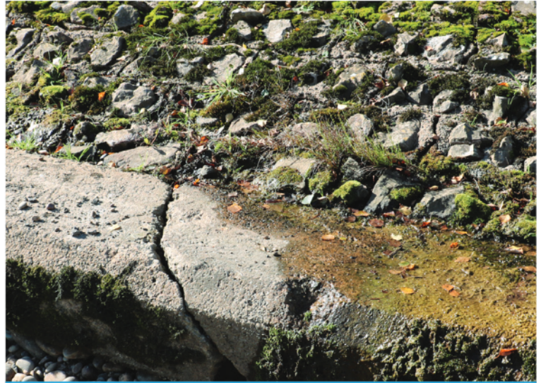
An area of the concrete curb which had badly cracked
